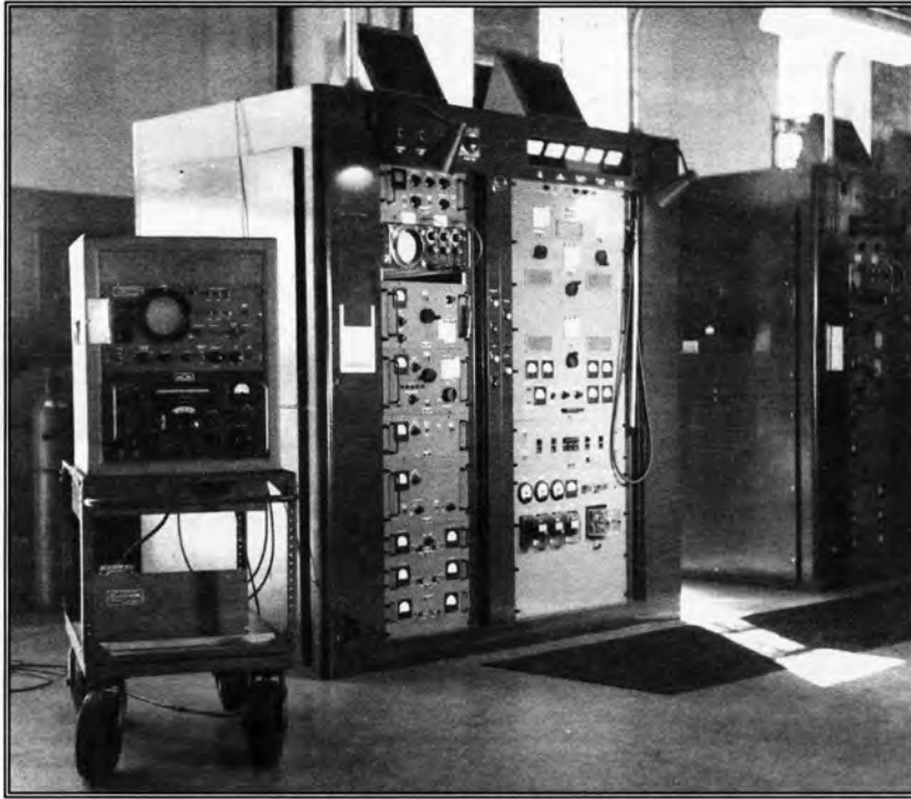
RCA developed and built SSB-T3, Type H Transmitter, Single Sideband, 20 kw P.E. 17 at Rocky Point.
